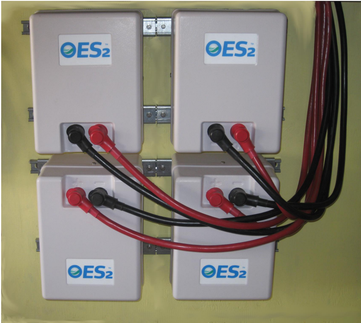
Figure 1.5 Four OES 2 ™ 48V Modules Mounted on Strut Rails.
